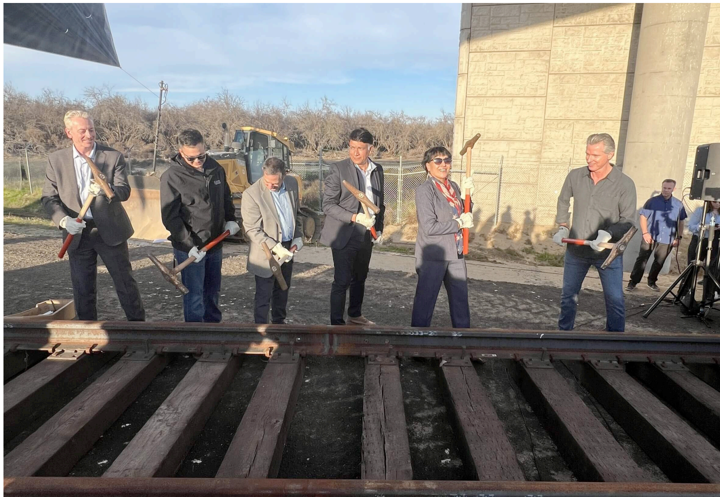
Governor Newsom, CEO Choudri, partners, and community leaders pound spikes to kick-off the Railhead Project.
